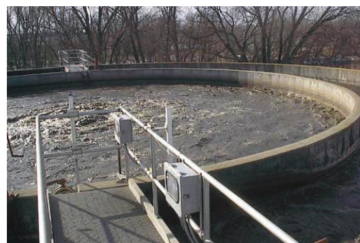
A waste water treatment plant
